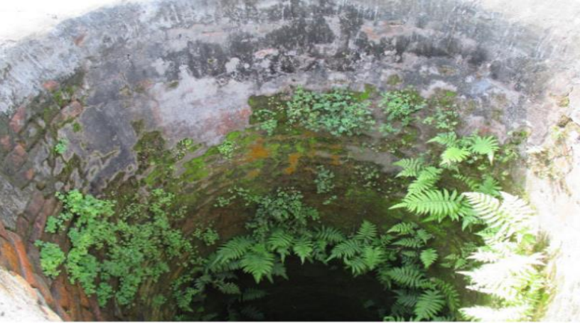
Well before maintenance
